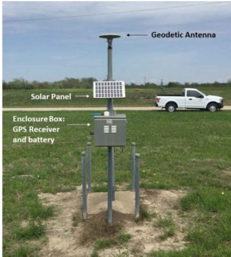
Figure 4-6 Example of a complete subsidence monitoring station with all geodetic instrumentation and power supply equipment installed.
